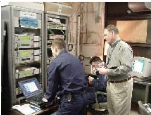
Loran-C; installing a receiver [ https://goby.nrl.navy.mil ]
